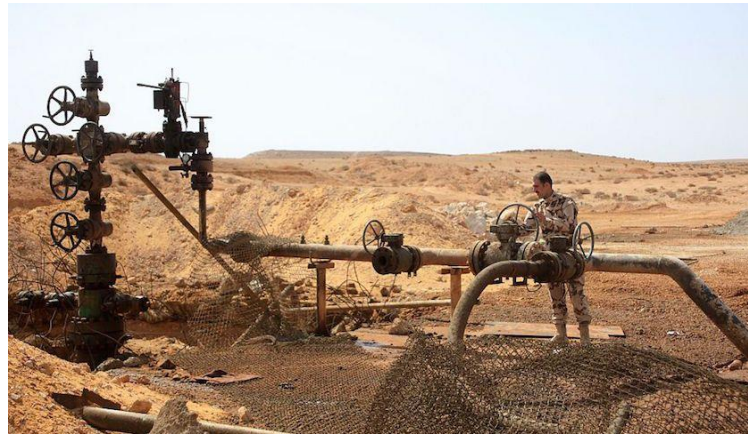
Picture 1 – Old worn-out wellhead in one of Yemen's oilfields with damages caused by bombings
